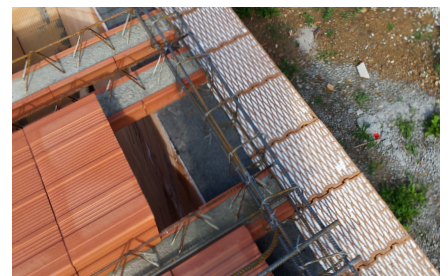
A bitumen band of at least 3.5 mm is applied only in the ceiling support area and the future reinforced concrete ring beam!
