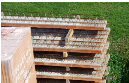
Check the material delivered according to the assembly drawing – type, dimensions and number of ceiling girders, panels and capping course blocks.
